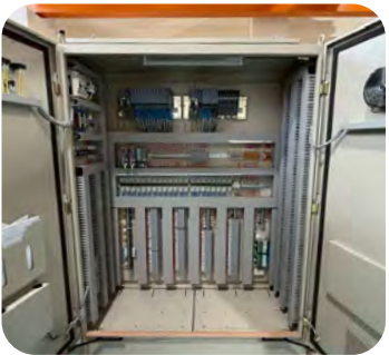
Mixed acid equipment redesigned to use DC power
