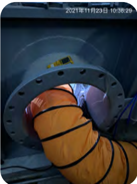
Continuous Ventilation and Air Exchange
