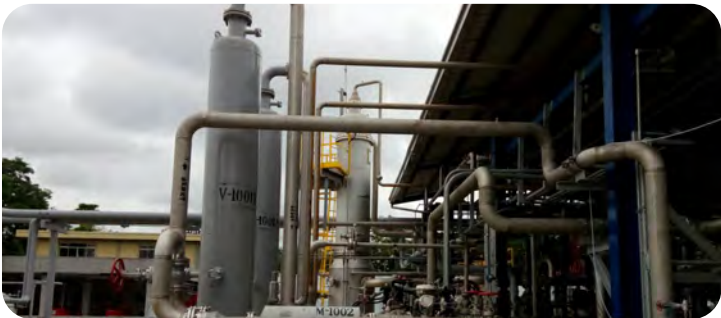
Membrane Vapor Recovery Equipment
