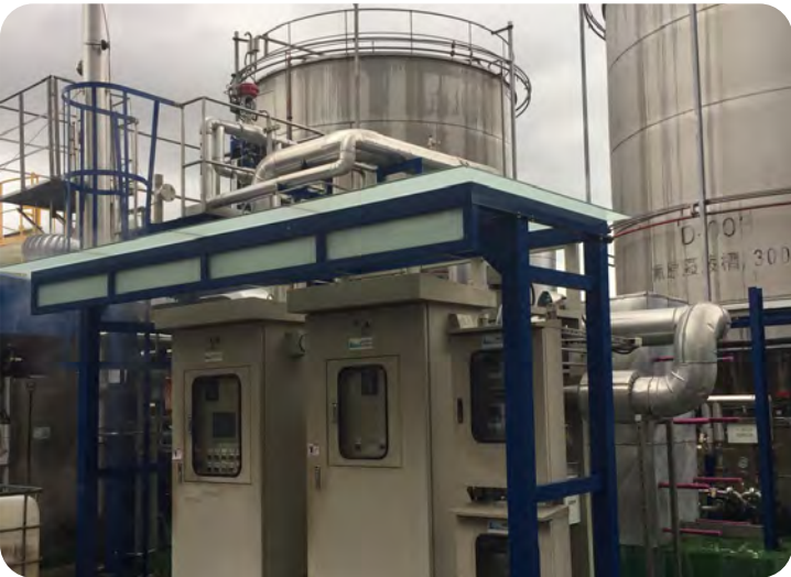
Chemical Waste Liquid Recovery and Reuse Equipment
