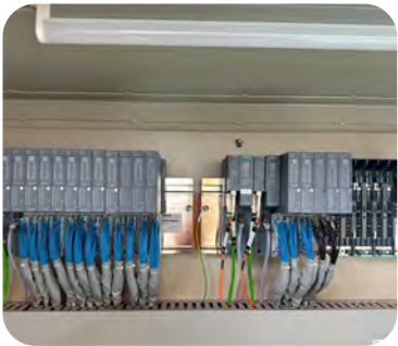
Machine lighting changed to energy-saving fluorescent lights (5W)
