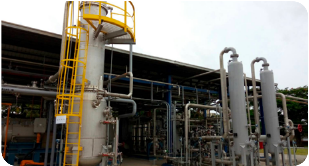
Membrane Vapor Recovery Equipment
